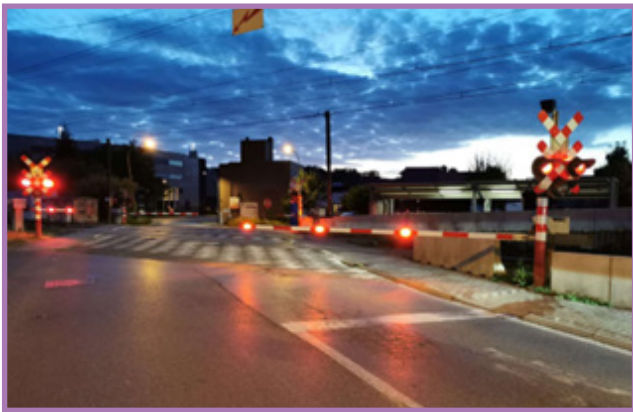
Figure 30: Barriers with LED lighting. Source: (Infrabel, 2024d)
